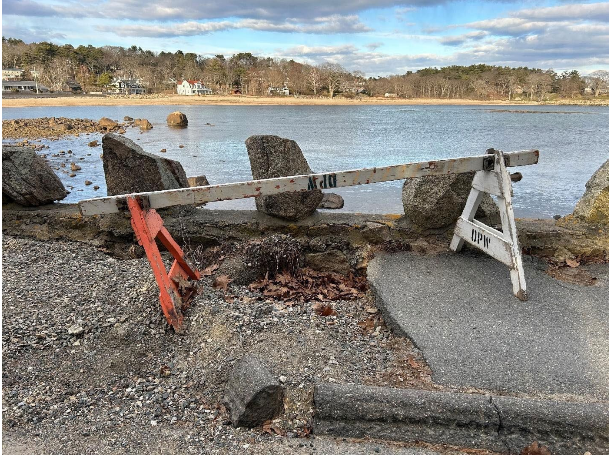
Figure 21: Crumbling pavement near White Beach.
